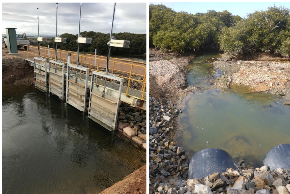
Figure 5. Tidal gate infrastructure showing the controllable gates (left) and the polyethylene pipes connecting the trial pond to pumping creek and mangroves in Barker Inlet (right). Photos L. Mosley and S. Dittmann.
